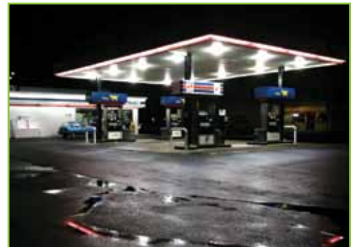
After Metrolight 250w SmartHID™ electronic ballasts - maintained lighting levels
