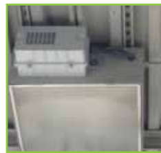
After Metrolight Metrolight's 200w EcoBOX for the Canopy Lights
