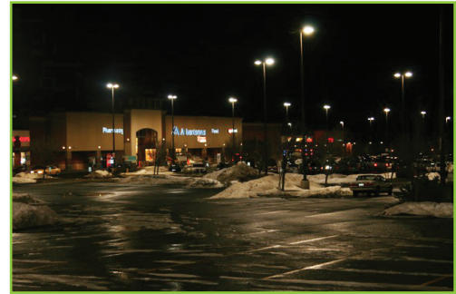
Before Dimming 1000W MH shoebox fixtures on 40' poles
