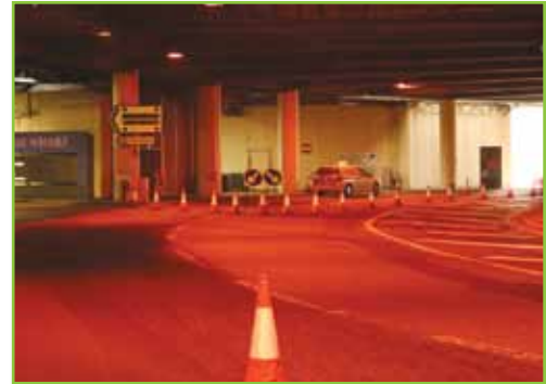
Before Metrolight 400W Standard Gear
