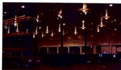
UK Grocer Distribution Center Before Metrolight: 400W HPS Luminaries
